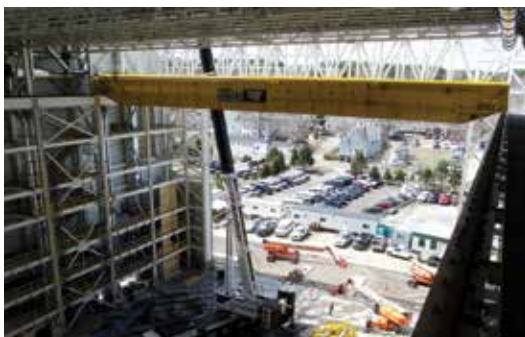
8. The East Crane ready to receive its two trolleys, each with a 100-ton and 25-ton hoist.
