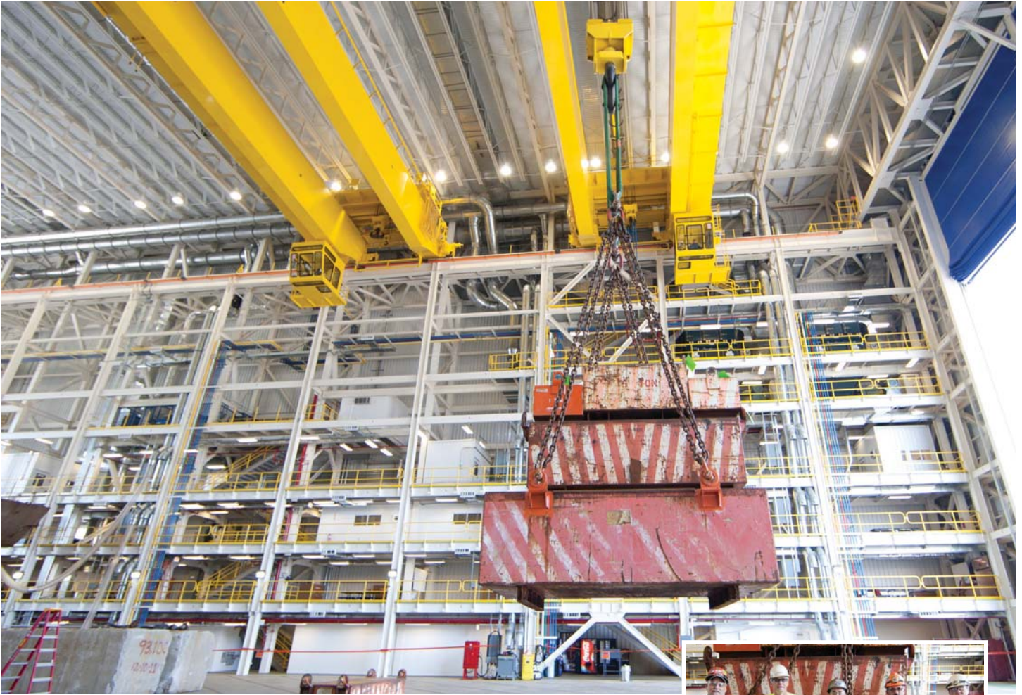
A 30-ton test load is suspended from the West 200-ton bridge crane during the installation and testing phase of the Outfitting Hall cranes.
