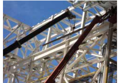
3. The crane runways were installed with part of the roof open to accommodate the 550-ton crane which would raise the girders 83 feet aloft. The installation was staged in West Bath.
