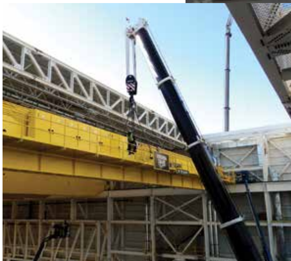
9. With the last girder of the West Crane landed, all four girders were in place.
